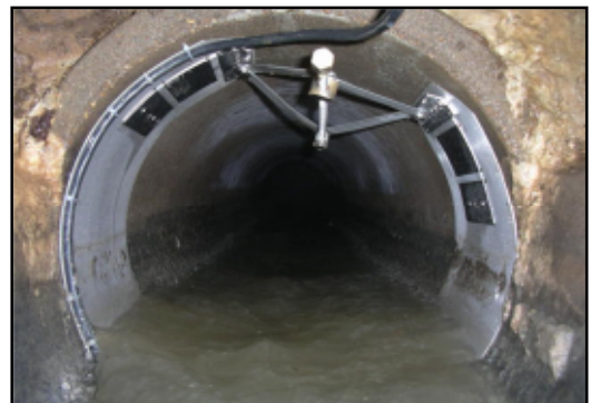
Exhibit 2: Flow Meter Installation
